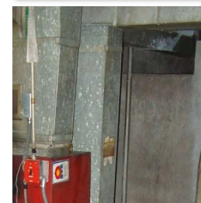
Broken ducts = higher heating bills
