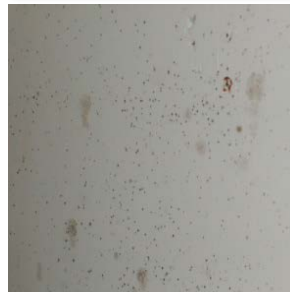
Water leaks = mold hazards
